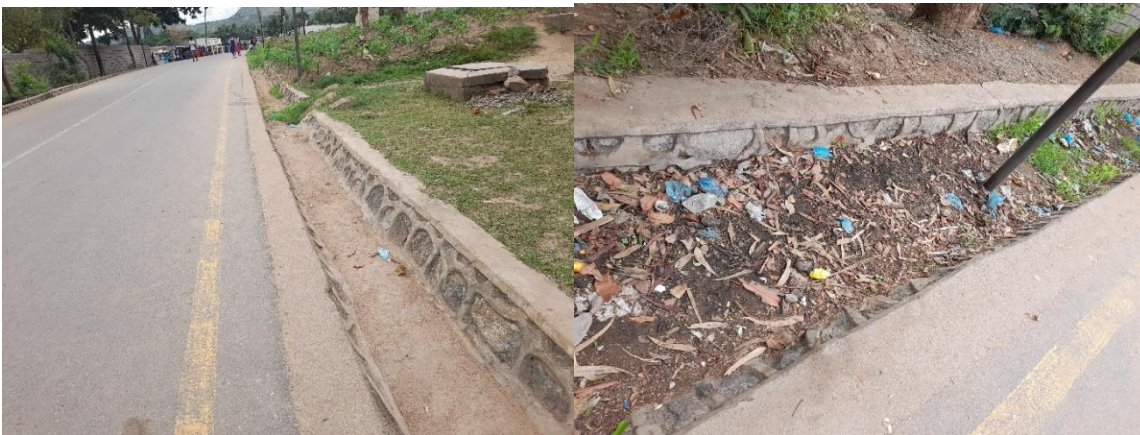
Figure 8: Showing Luwanda to Namilango school road condition which was upgraded in 2018 Source: Author's capture
