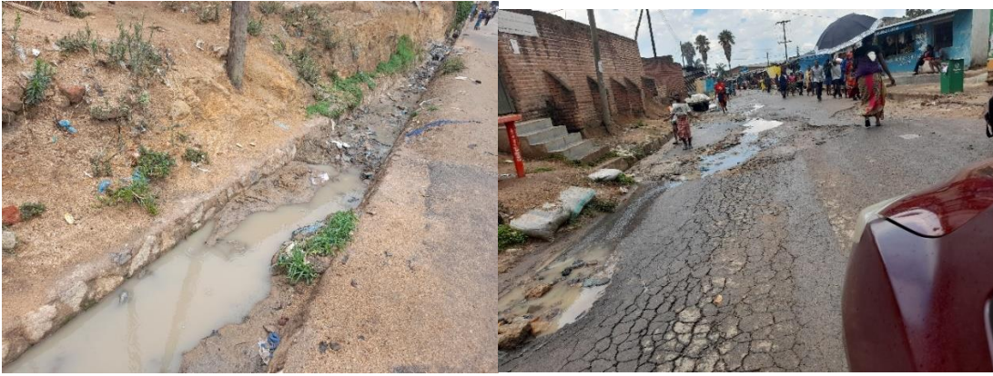
Figure 7: Showing the Safarao road condition which was upgraded in 2017 Source: Author's capture
