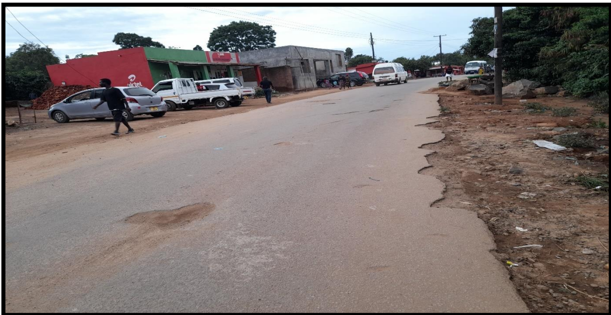
Figure 5: Bangwe to St.Patrics road with poor shoulders and without drainage system
