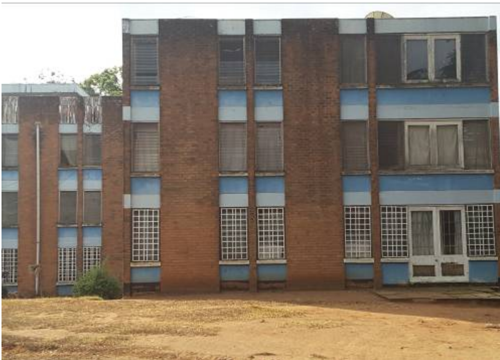
Housing estate window fittings also made of timber and exposed to outside environment
