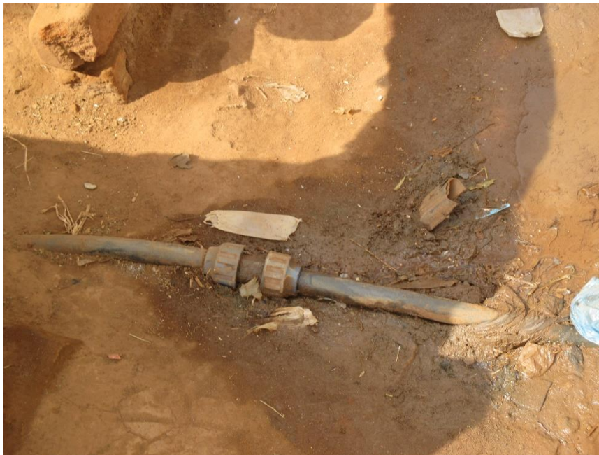
Figure 4-12: A leakage on an exposed pipe at Mgoni
