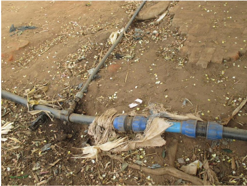
Figure 4-11: An exposed pipeline prone to vandalism and damage – Mtandire
