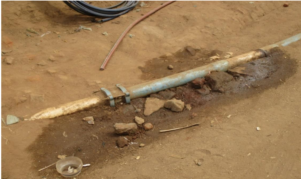
Figure 4-20: Visible leakage along a main road at Mtandire
