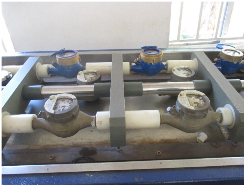
Figure 3-3: Meter testing at the meter laboratory
