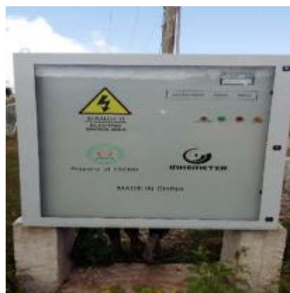
Figure 10: Energy consumption meter.
