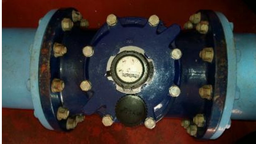
Figure 9: Pumping station flow meter.
