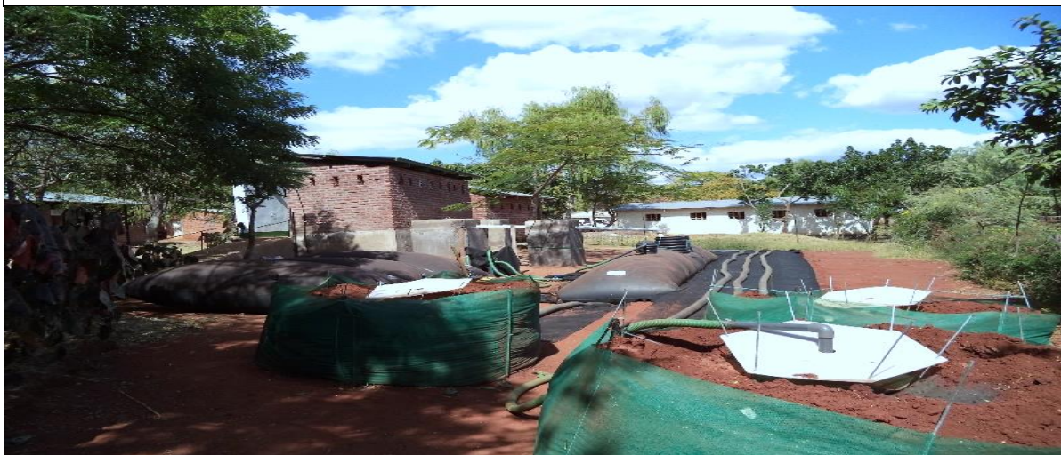
Figure 15: Anaerobic Digester Connected to Pour Flush Toilet
