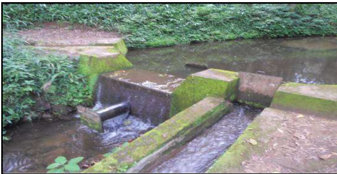
Figure 29: Livingstonia GFS Water In-take at Nyankhowa Stream
