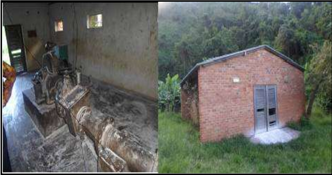
Figure 27: Hydro-electricity Plant Powered by Scheme Water from the Reservoir Tank
